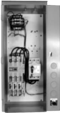
Irrigation Pump Panel
