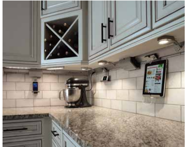
Under-Cabinet Lighting System installed in a kitchen.
